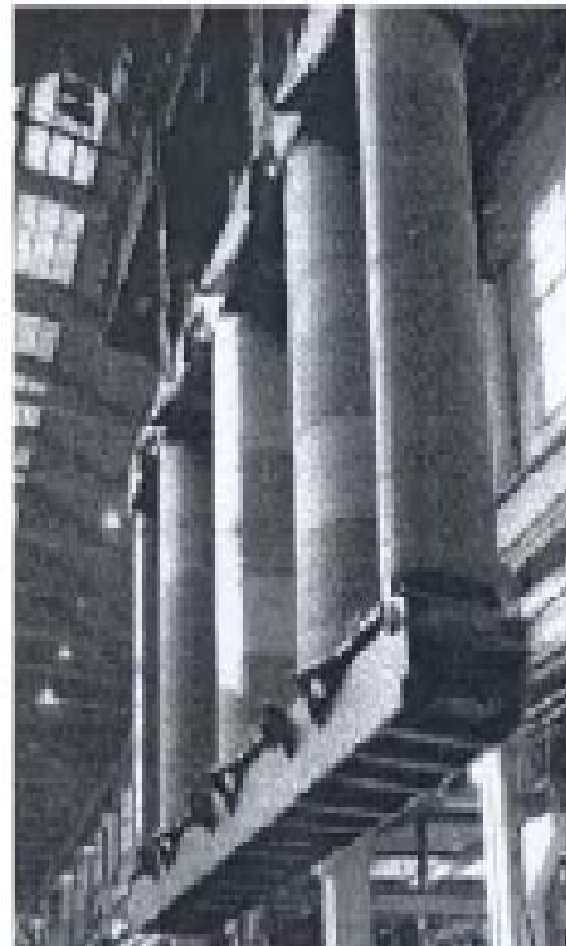
Figure 10 A photo of a shell-type three phase transformer.
